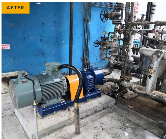
EHIK pitot tube pump · production lines 1 and 2
