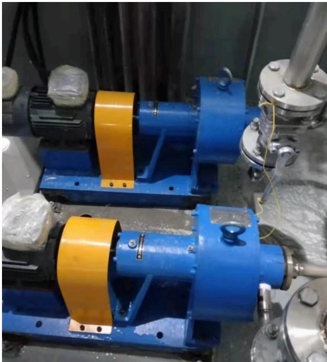
EHIK pump sets serving the water-needle cutting application at Xiawang Paper.
