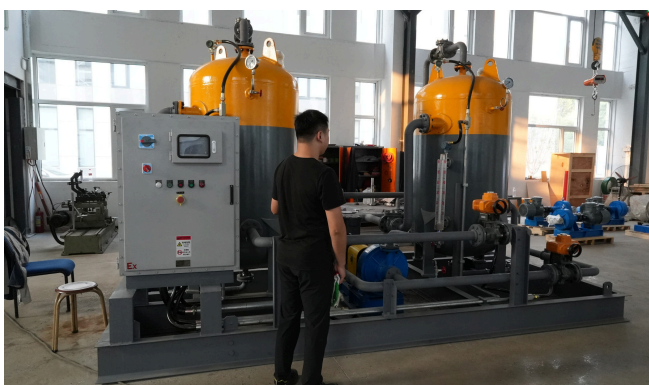
Complete skid at EHIK.
