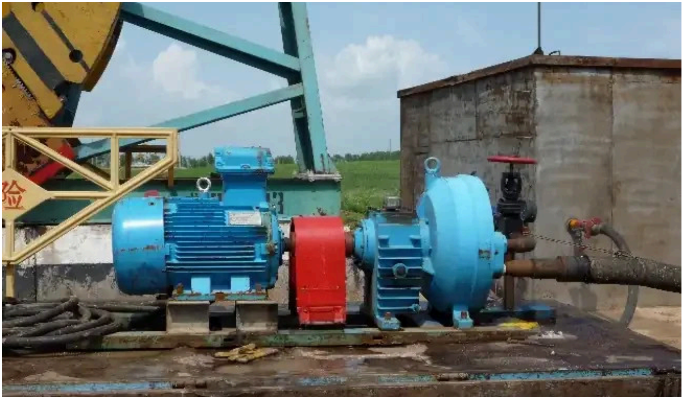
Hot-water well-cleaning installation at Longhupao Oilfield, 2010.
