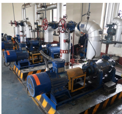
Naisiter · Connected pump and drive
