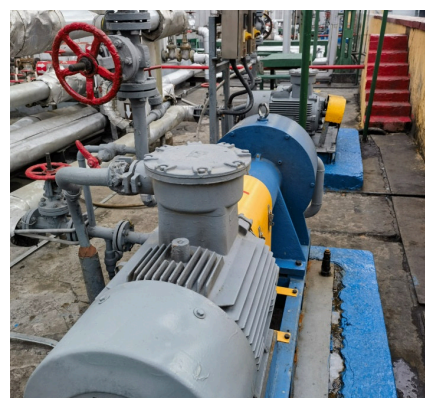
Longxing · Plant equipment
