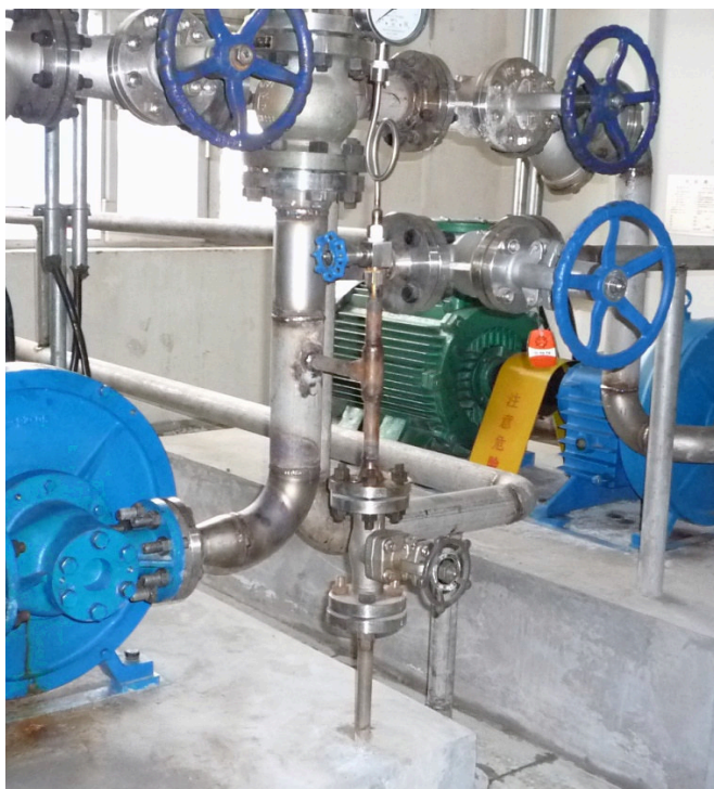
Daqing synthetic ammonia workshop — EHIK pump
