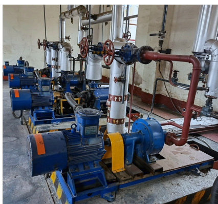
Naisiter · Feedstock- and fuel-oil pumps
