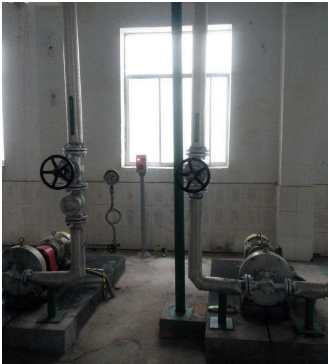
Rongxian purification plant — hot-water pump
