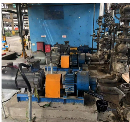
Yunwei Feihu · Pump and pipework
