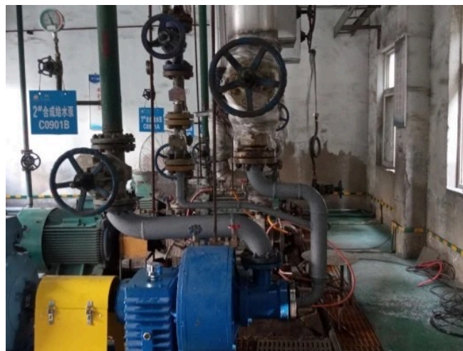
A closer view of the pump, drive and process connections.
