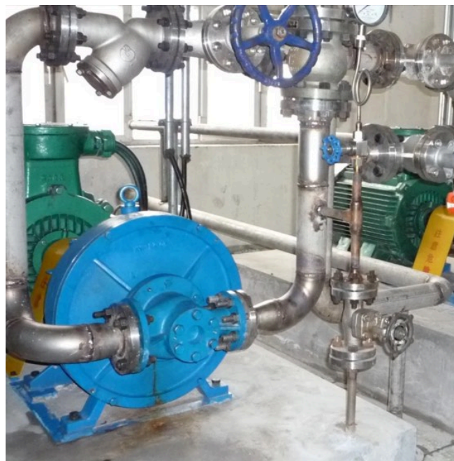
Synthetic ammonia workshop · the EHIK pump that replaced a 75 kW (101 hp) multistage pump in 2010.
