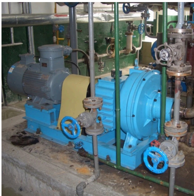
Methanol workshop · EHIK pump in service after the 2009 replacement.
