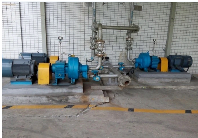
Shower-pump installation with the surrounding pipework and valves.
