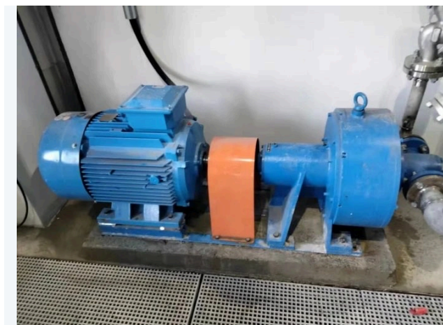
A separate EHIK pump serving the mill's flushing-water circuit.
