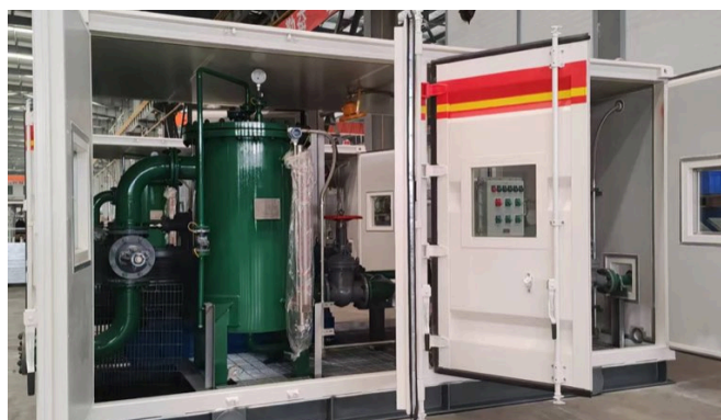
Doors open for access to the pump, pipework and controls.
