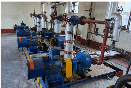
Naisiter · Feedstock- and fuel-oil pumps
